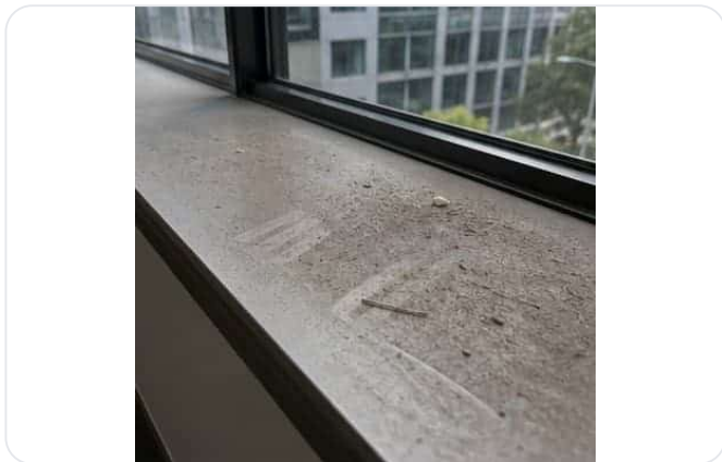
Dust build-up on office window ledge before service
