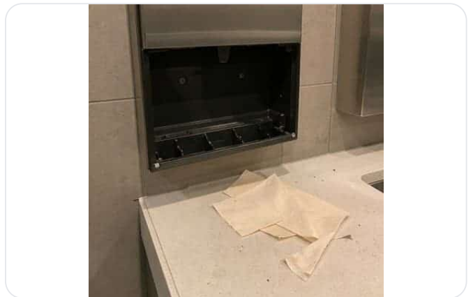
Restroom consumables low before restock
